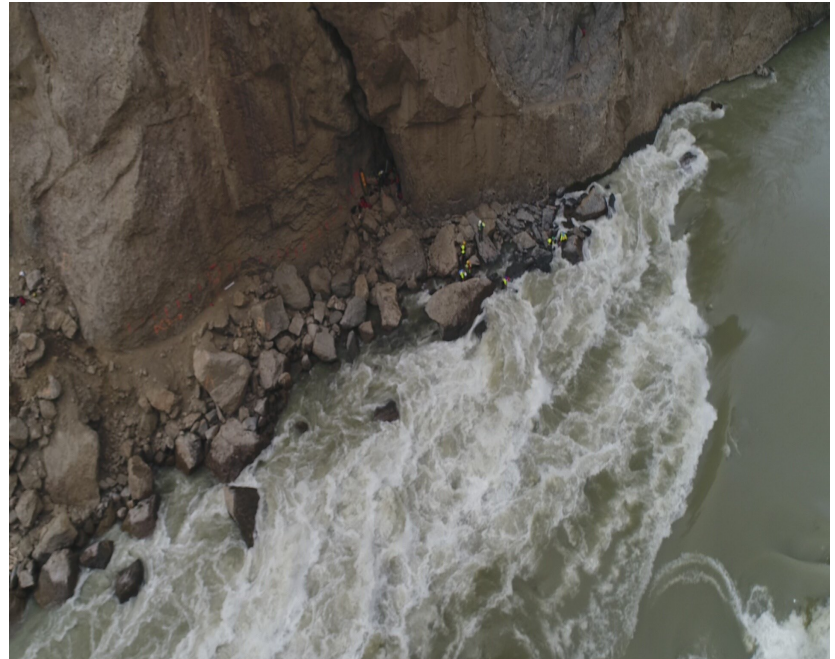
Rock scaling crews conducting rock manipulation to create pools and passageways (along the shoreline) for natural fish movement upstream.
